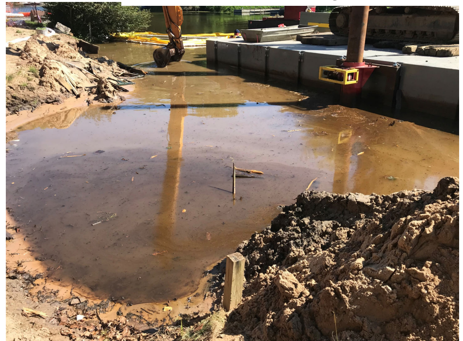
Observed Oil During Excavation
