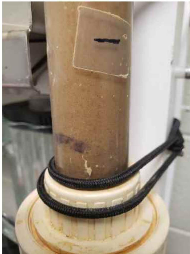
During CLEAN injection and backwashing
