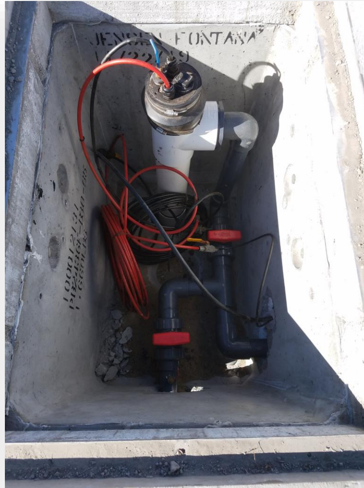
SVE Wellhead (Newly Installed)
