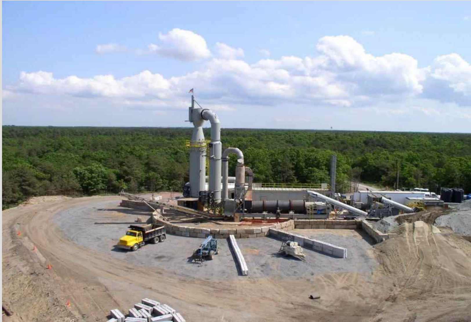
Photo of TDU to be Utilized
