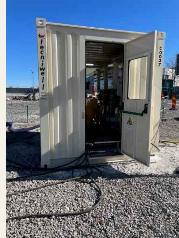
Automated pump station allowing for injection at multiple points simultaneously
